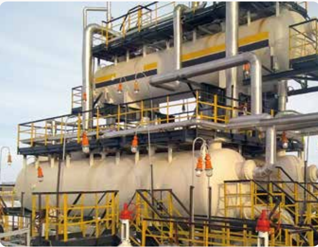
< GOSP (Gas & Oil Separation Plant) >
